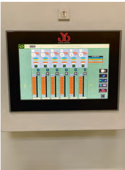
JB Machinery Control Panel
