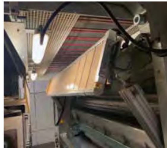
JB Machinery dryers fitted to the new Ovation
